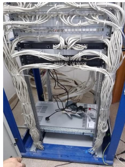
Screenshot 2 Data Center upgrade – Switches, Gigabit Ethernet Server, optical fiber
